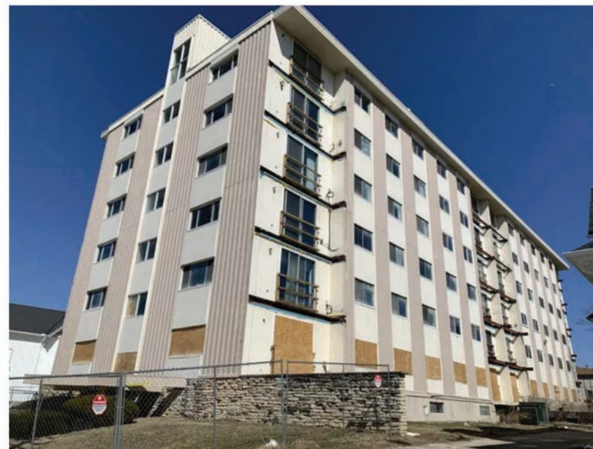
The Horizon West Condominiums building stands vacant and partially boarded up in late March 2023. The building's owners remain in limbo, with their assets tied up in the structurally compromised building, as they continue to seek relief from their insurance company in court. Jim Riccioli / Now News Group
