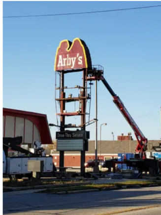
The Arby's sign in Cudahy was taken apart Nov. 1, 2022 after the business closed on Halloween the day before. Submitted By Mike Tichkowski
