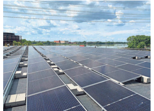
More than 400 rooftop solar panels generate electricity atop Kimberly-Clark Corp.'s Experimental Mill in Neenah. COURTESY OF KIMBERLY-CLARK CORP.
