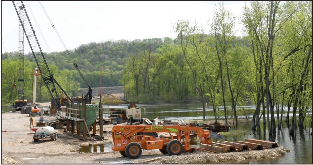
KRAMER CONSTRUCTION has resumed work on the north end of the Lone Rock Bridge replacement work site. High water can once again be observed as the Wisconsin River responds to precipitation events in the upper parts of its basin, but nowhere near levels seen a few weeks earlier.
