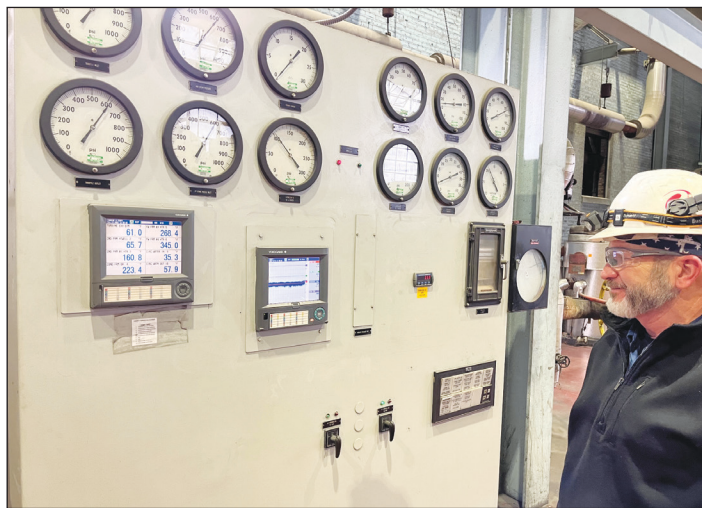
Gauges near the turbines keep track of operating temperatures and generator output. (Peter J. Wasson/Staff photo)
