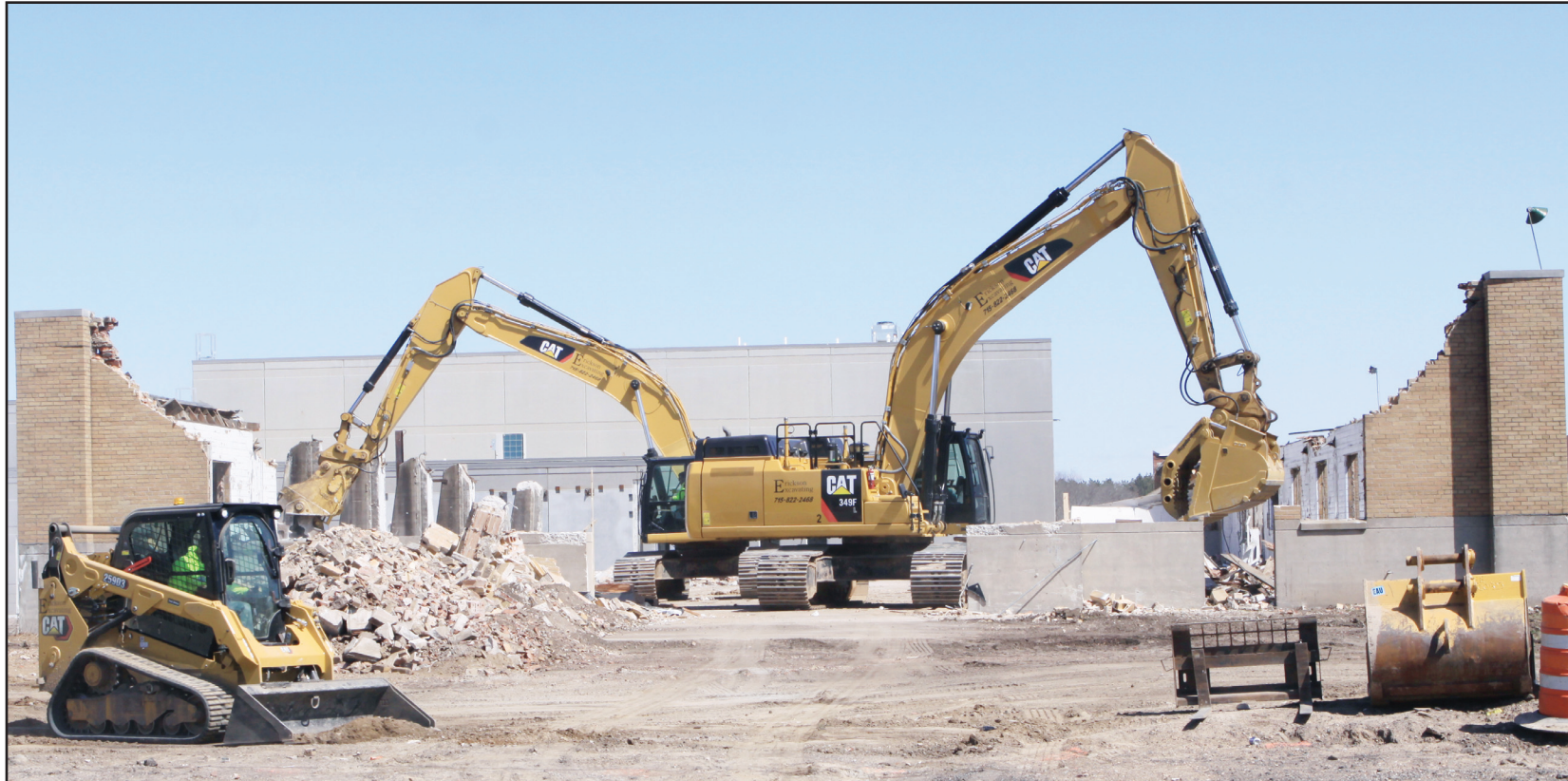
Highway Shop is history — Crews from Erickson Excavating completed the demolition of the former Barron County Highway Department shop this past week. The old shop was designed by E.F. Klinger and Associates, of Eau Claire, and constructed in 1947 on the east side of Hwy. 25 by Peterson Construction Co., of Minneapolis, at a cost of $191,000. Citing needs for modernization and more space, Barron County elected in 2021 to build a much larger shop and other buildings. During that process, it was discovered that the 1947 highway shop was flagged as eligible for Register of Historic Places in 2011 by the Wisconsin Department of Transportation. The discovery delayed the project and contributed to the cost rising from an estimated $25 million to $30 million. Once the debris is cleared, the area will be used mainly for parking. There will also be a sign and display recognizing the history of the shop that stood before. Photo by Ryan Urban
