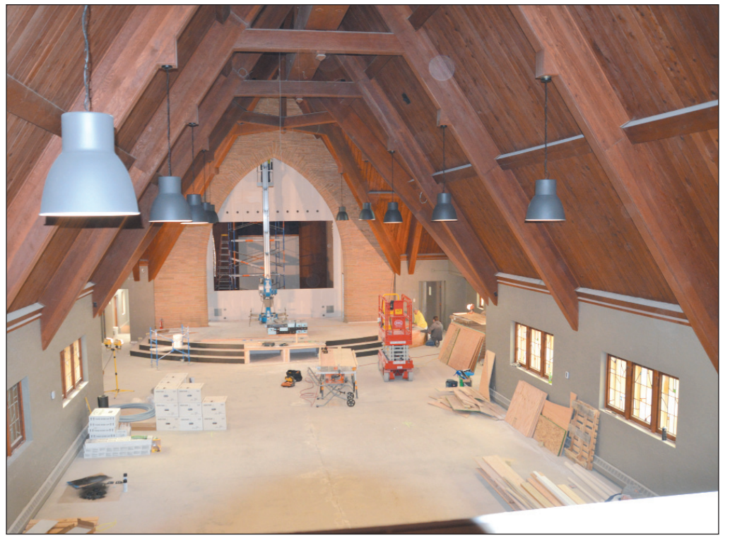
The interior of the former St. Matthew's Church is being updated to have a more modern look, but some original features like the stained glass windows will remain.
