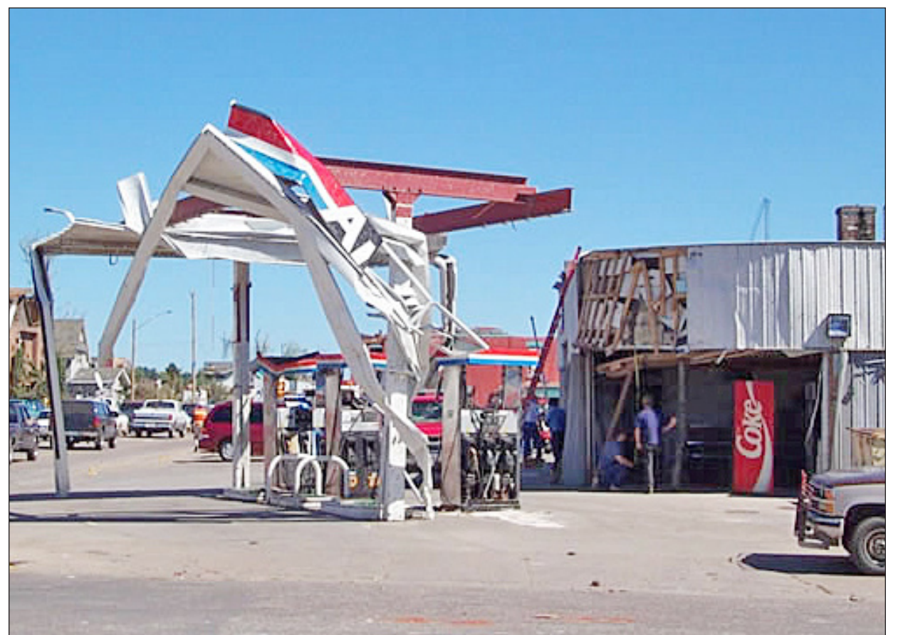
STATION DAMAGED — Jerry's Amoco is severely damaged. The station's fuel island canopy is destroyed, and the shop has siding torn off.
