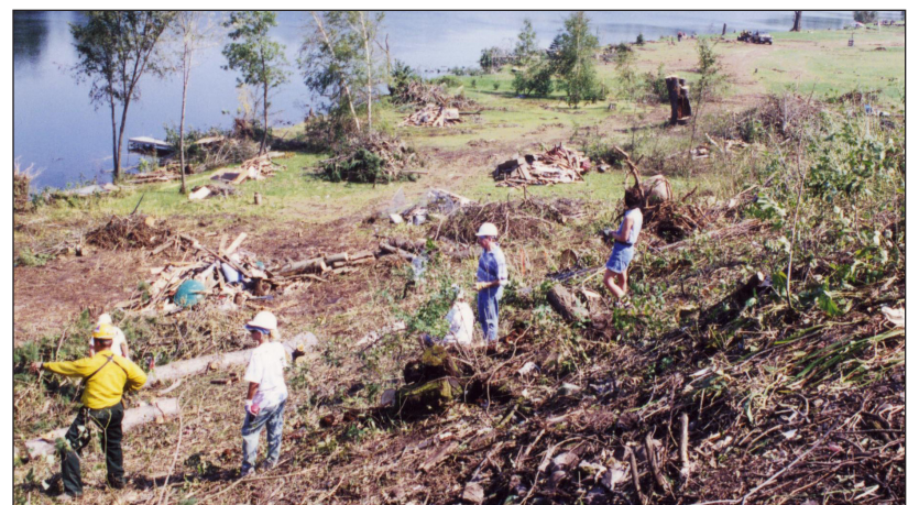
CLEANUP BEGINS — Crews survey the damage on the south shore of the Flambeau River. Since then, this area has grown over with vegetation.
