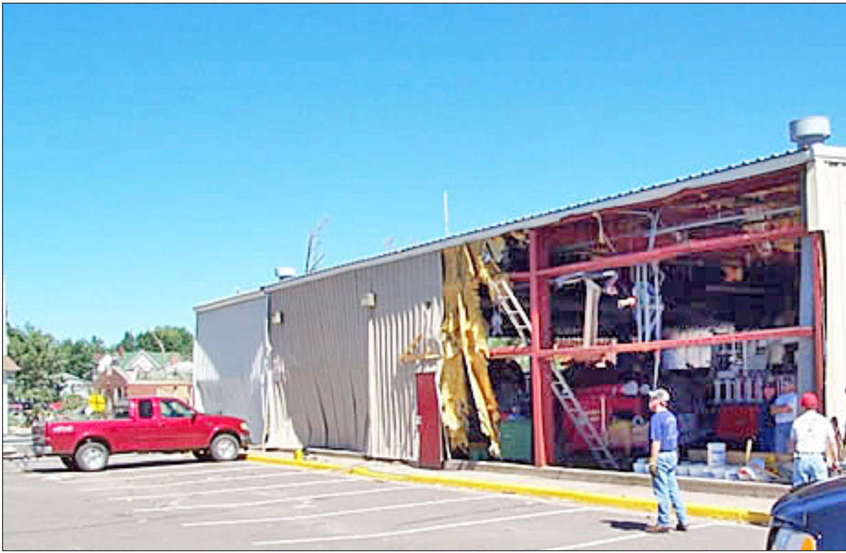
EMERGENCY REPAIRS — Siding is ripped off the old fire hall southwest of the intersection of Miner Avenue and W. Third Street, exposing fire trucks and other emergency vehicles to the elements.
