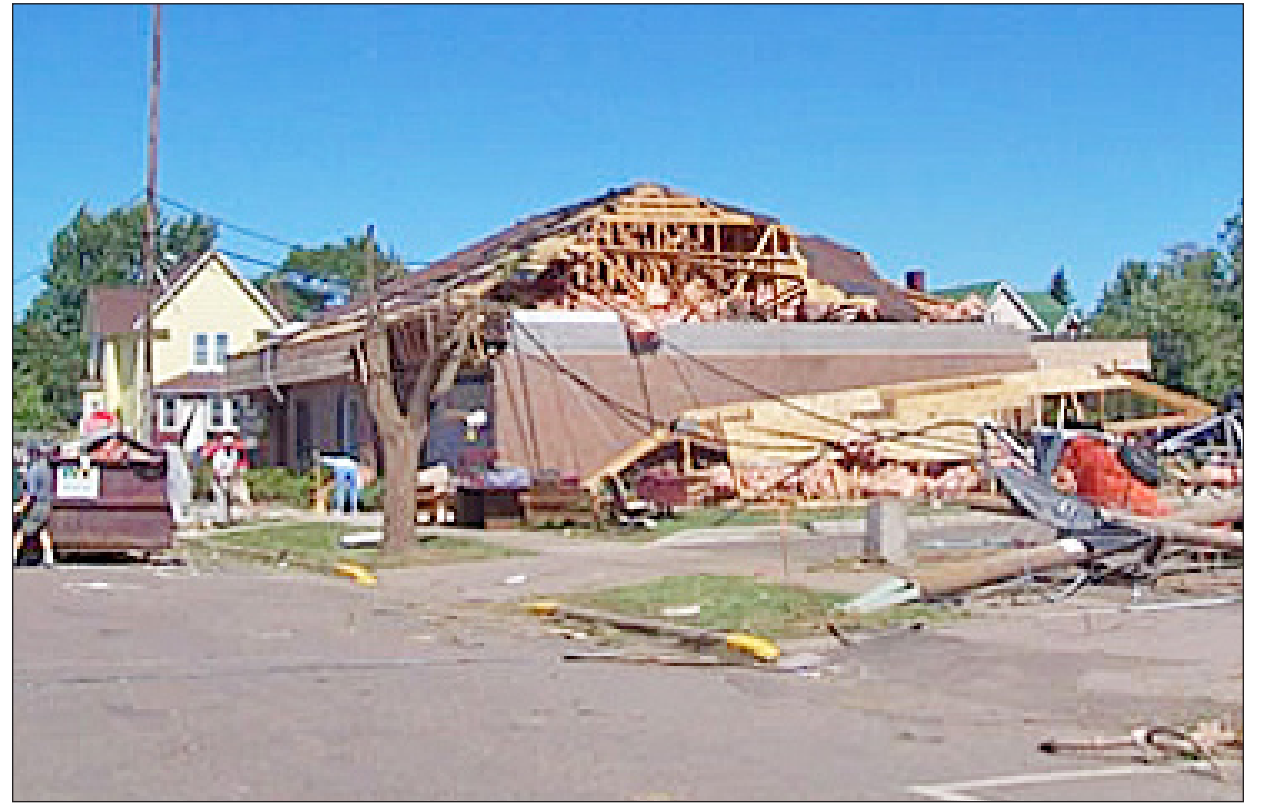
ROOF DAMAGE — The Ladysmith Federal Savings & Loan building along Lake Avenue, southeast of W. Fourth Street N, takes on massive damage as its roof caves in.
