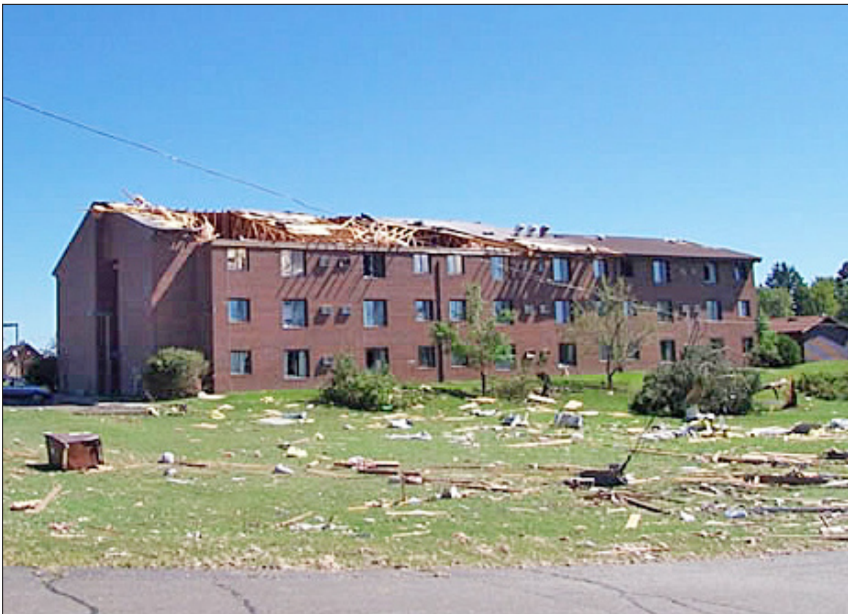
APARTMENTS DAMAGED — Greenwood Manor Apartments along Miner Avenue east of Wis. 27 is heavily damaged as parts of its roof it torn off.
