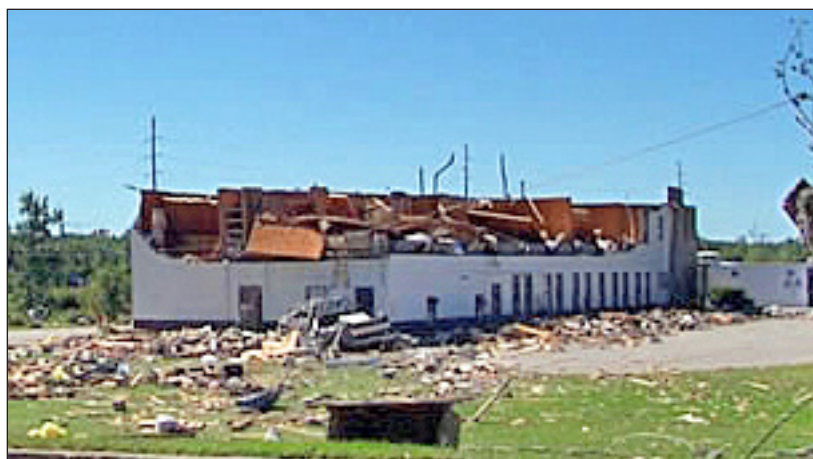
SHEERED OFF — The upper floor of the former Davis Motel in Ladysmith is exposed to the air during the storm.
