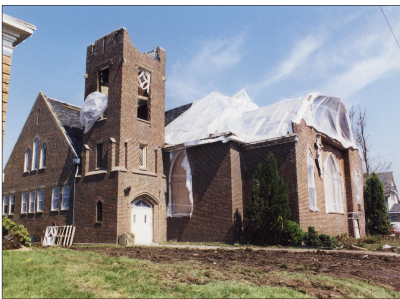
OPEN AIR MASS — Plastic sheeting is used to shield the UCC Church on Lake Avenue from the elements after the structure was severely damaged.
