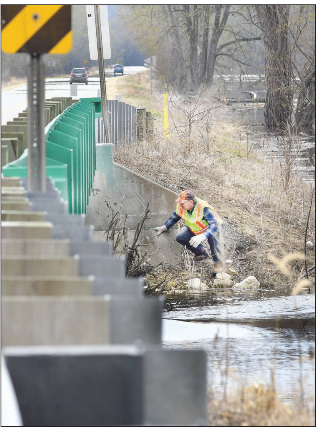
A WISCONSIN DOT EMPLOYEE inspects the structure and flooding at one of the small bridges along the Lansing Dike on State Highway 82 on Monday afternoon. Rushing water in this area a few years ago undermined the dike below the pavement resulting in the fatality of a motorist whose vehicle was sent crashing to a whirlpool of water adjacent to the dike. As waters rose due to the flooding, the WDOT decided Tuesday morning to close the dike to all traffic until the flooding abates and the structure of the dike can be reinspected for safety.
