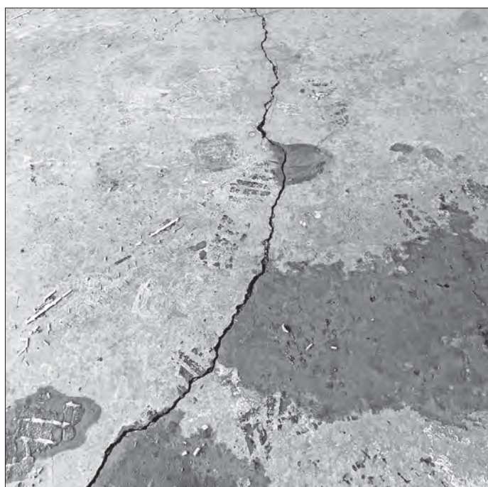
Homeowner Jon Wagner alleges that cracks such as this one to his foundation are a result of the deconstruction project. —Contributed Photo
