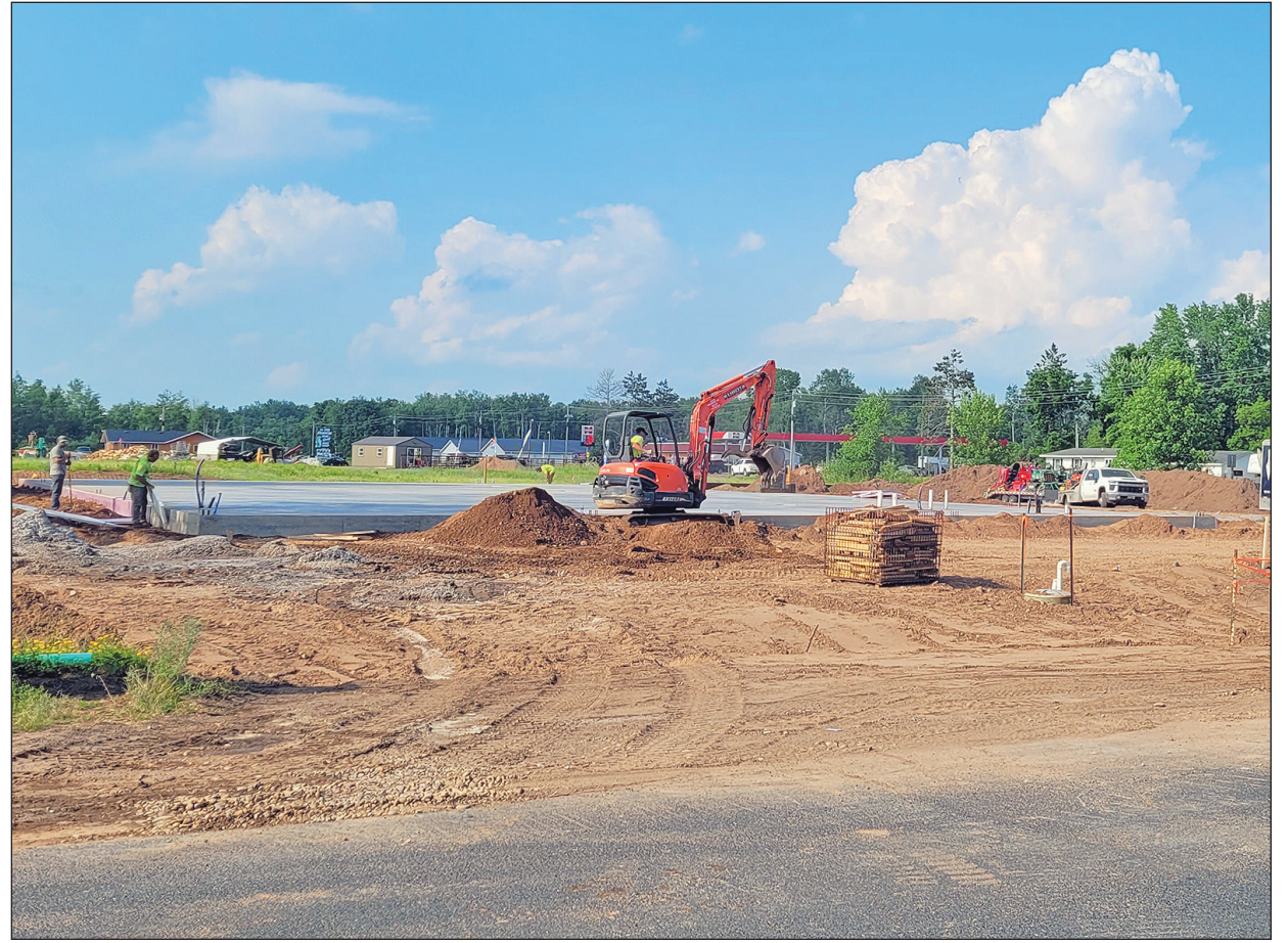
COMING SOON — The foundation is completed for the new Dollar General store being constructed in Holcombe. The new development on a 2.07 acre site is at the northwest corner of Wis. 27 and 263rd Ave., roughly across the road from Meadow Creek Mall. Plans call for about a 10,600 square foot building with 6-10 full time employees. There is highway access to the property, slightly north of and across from the mall driveway. Town Chairman Brian Guthman said state plans for site and driveways were all approved. He added owners plan to open this October or November. — News photo by Luke Klink
