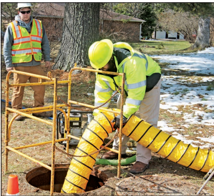
Utility locators Jordan Cook (left) and Will Scoins of the U.S. Infrastructure Corporation worked to find and test communications cables in Eagle River. —Staff Photo By JON EICHMAN
