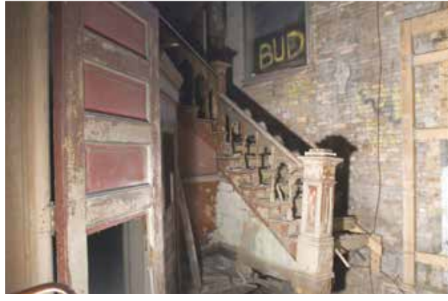
The original stairway with rubble and exposed brick at the Menominee Opera House.
