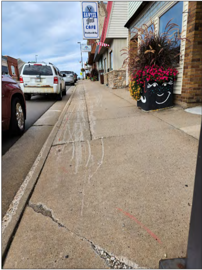
This portion of sidewalk, extending from the new library at 388 W. Main St. to Chestnut Street, is one segment that will be replaced by Pember Companies. Photo by Sarah Nigbor
