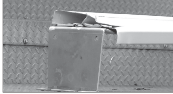
Broken bleacher seat at Preble High School.
