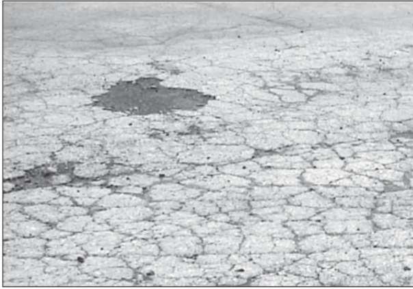
Stadium asphalt damage at West High School.
