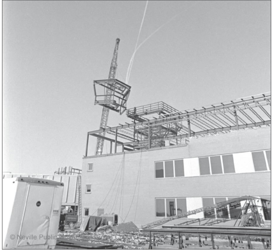
The frame for a six-sided glass observation cab is hoisted to the top of the observation tower skeleton in 1972. The observation tower was built to be five stories tall.
