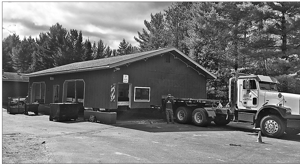
Merrill-based Schuette Movers ready 70 West Auto Body's original two-bay shop facility for its three-mile relocation to 628 Highway 17 South.
