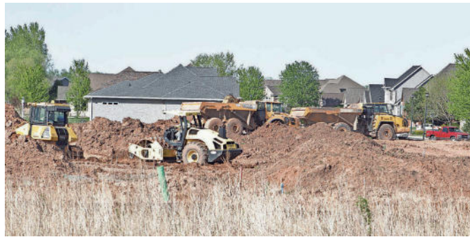
ABOVE: Crews prepare land for the next phase of a residential housing development on Wrightstown Road and East Frontage Road in Wrightstown.
