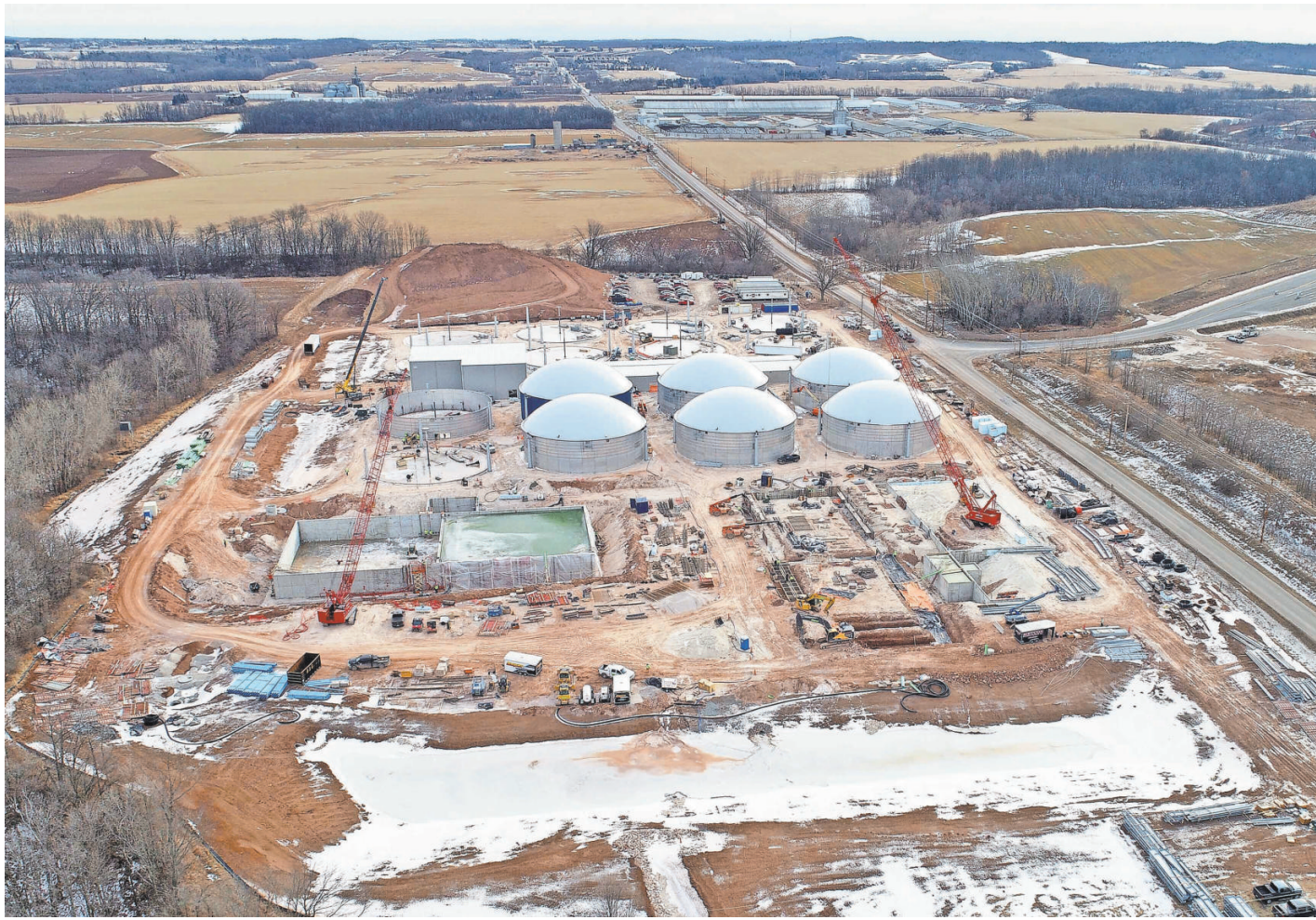
Construction of a dairy cattle manure digester facility is underway at BC Organics in Greenleaf. The Brown County plant will be one of the largest dairy cattle manure digesters in the nation and will process more than 360 million tons of manure a year into methane gas that’s put into a utility company pipeline. It’s scheduled to start operation this summer.
