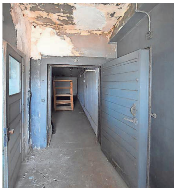
Third floor of the 1925 addition at the stair landing and entrance to cold storage room at Winnebago Cheese Factory.
