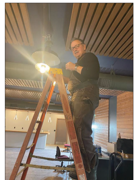
John Hunt of Hunt Electric installs lighting fixtures in the new Event Center. The center will seat up to 100 people for year around events. (Contributed photo)
