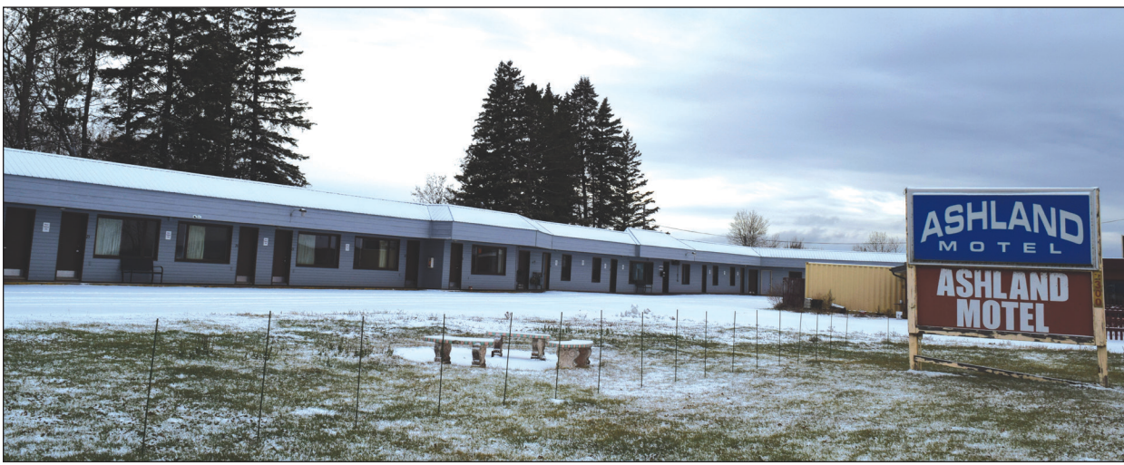
Organizers continue to renovate the old Ashland Motel to make it suitable for homeless residents who could be able to move in by the end of the year. (Tom Stankard/Staff photo)
