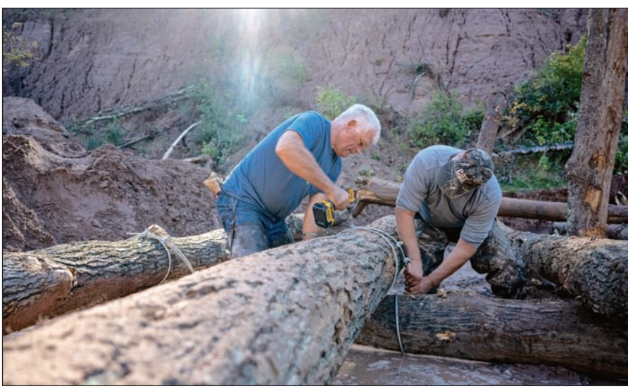
Work crews tie together logs with steel cables to form cribbing that will deflect the force of storm waters and reduce erosion on North Fish Creek. The project undertaken by Northland College's Mary Griggs Burke Center for Freshwater Innovation is one of several such efforts that will be needed to fully control silt runoff into Chequamegon Bay. (Contributed photo by Bob Gross)
