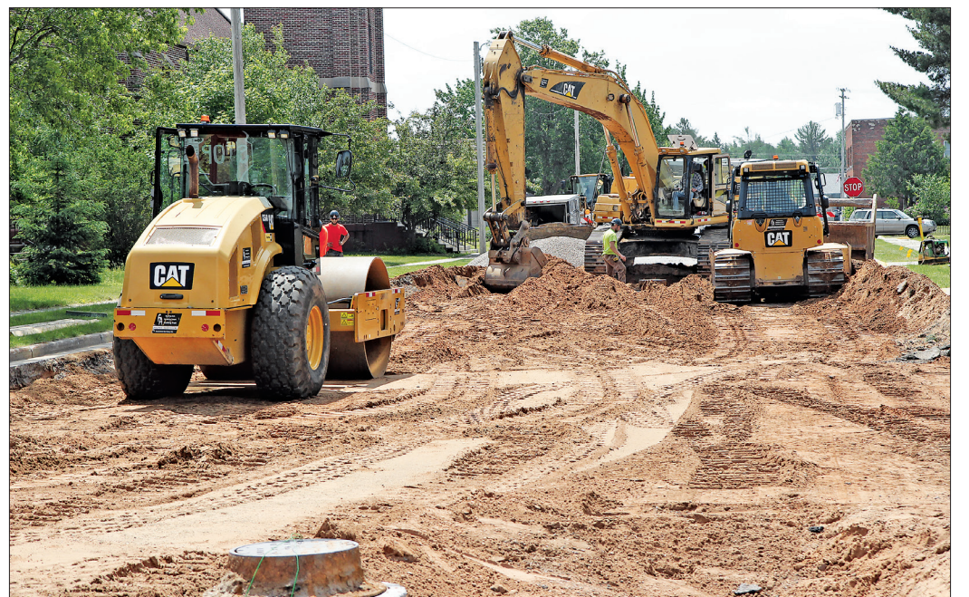
Road construction projects in the area have received another funding boost after the DOT announced recently that Vilas County would receive over $1 million. —STAFF PHOTO
