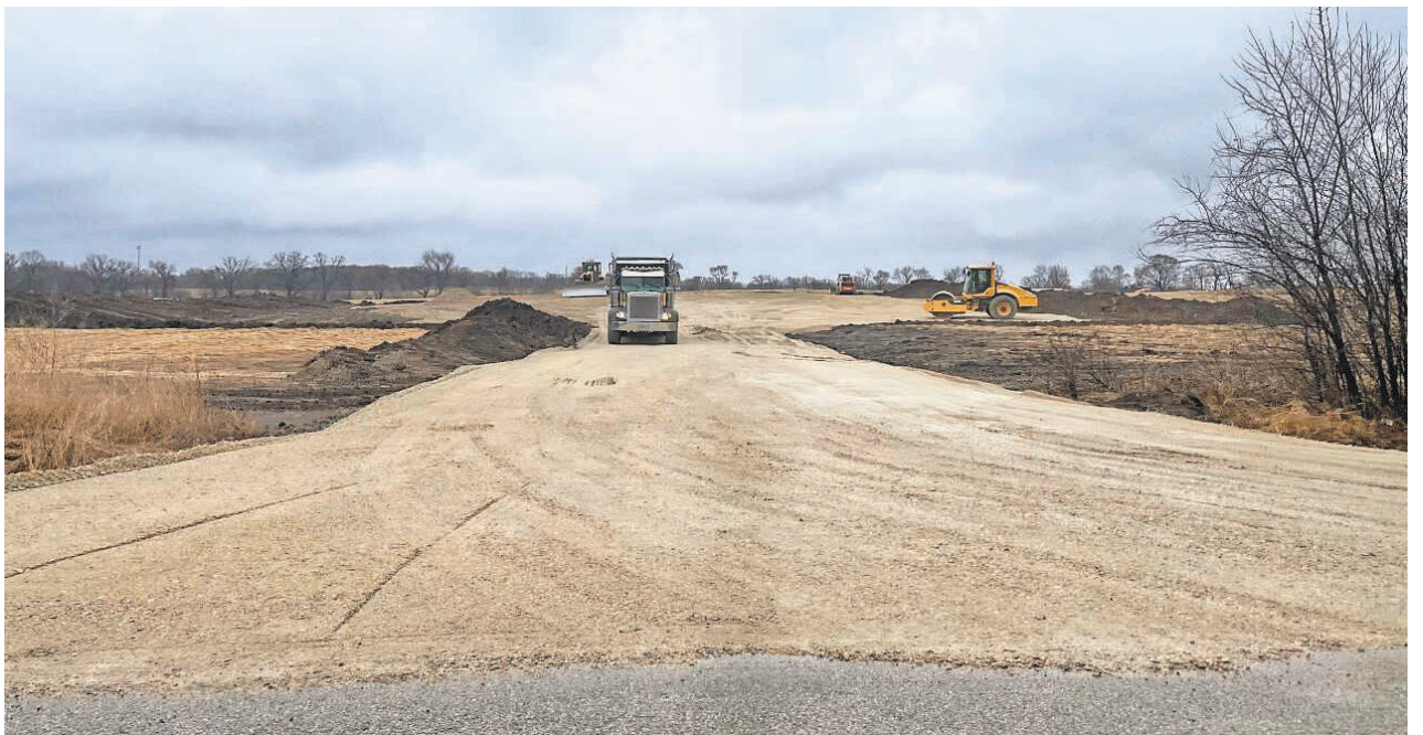
A dump truck moves along a newly constructed service road leading to a site that will be used to compost millions of laying hens impacted by the highly pathogenic avian influenza virus on a Jefferson County poultry farm. The land parcel, selected by the DNR, is owned by S&R Egg Company.
