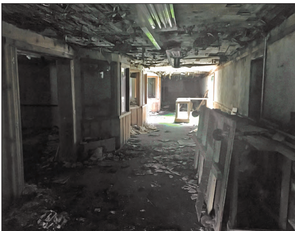
Fallen ceiling tiles, discarded display cases and other debris fill the ground floor main hallway at Eagle River's Big Barn Shops, where a carpet of moss now covers the old man-made
