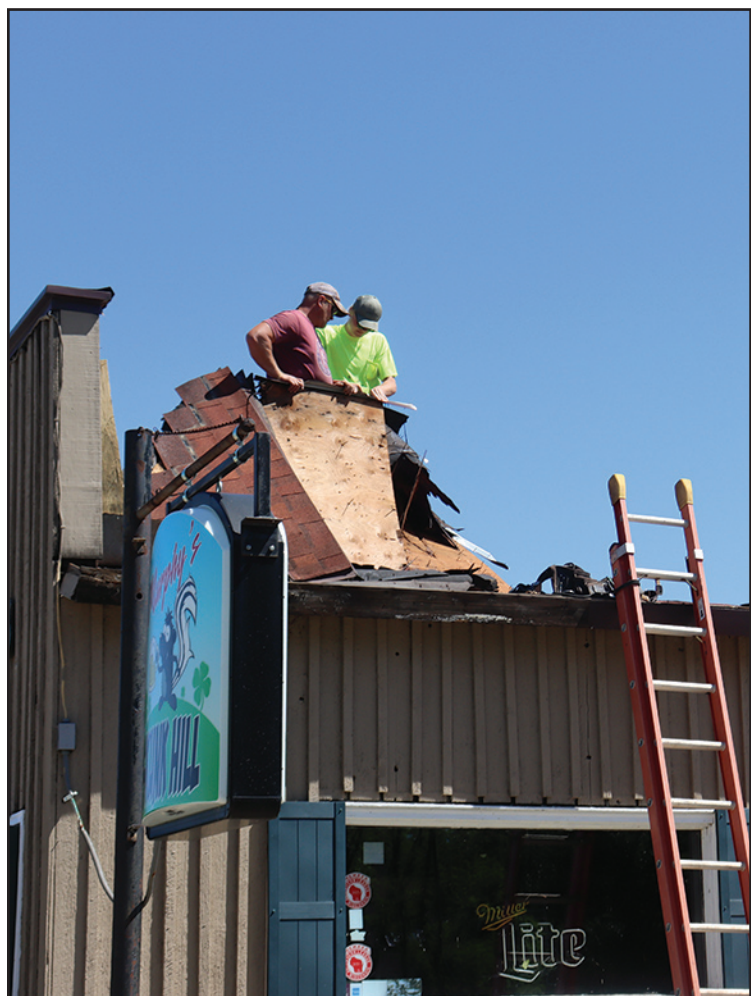
Workers from Brockman's Roofing and Siding were on the job June 16 right after the June 15 storm replacing the damaged roof at Skunk Hill Bar on Hwy S.
