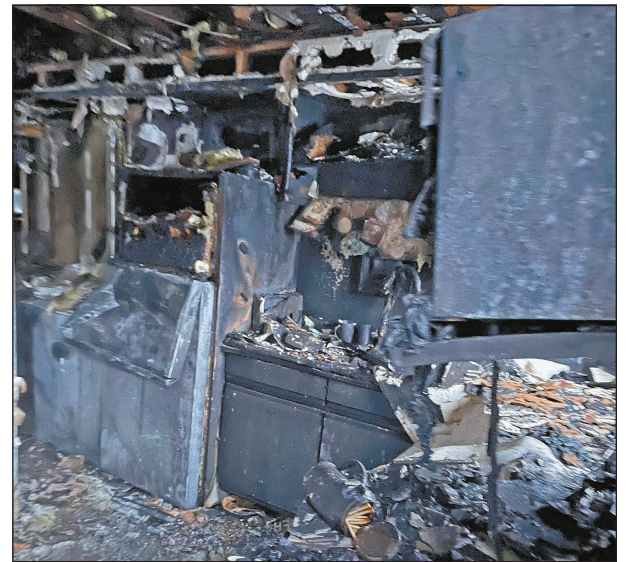
The interior of the lower apartment in one of the rental units at the Blue Haven Stables property is completely destroyed in a Jan. 13, 2022, fire. Submitted photo.
