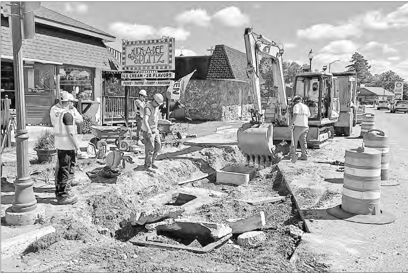
ROAD WORK — Major road construction projects continue in downtown Three Lakes, with crews replacing storm sewer inlets, and curb and gutters in preparation for the repaving of Highway 45 through the downtown area yet this summer and fall. Next year,
