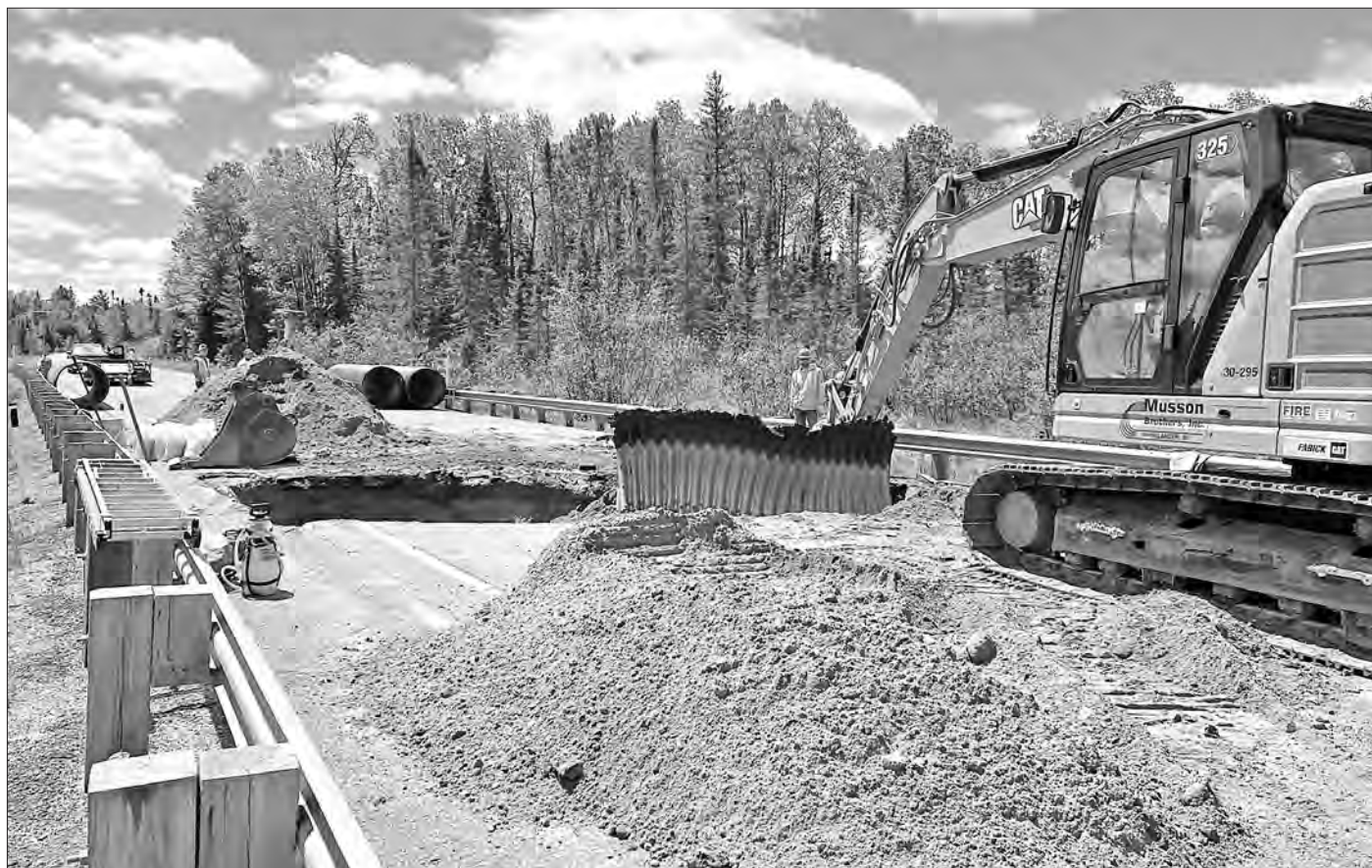
CULVERT WORK — Repairs were made the morning of June 3 to the Scott Creek culvert on Highway 32 east of Three Lakes. A
