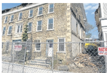
STEPHANIE JONES, REGIONAL NEWS Demolition began on Thursday, May 12, of East Troy's historic Cobblestone Inn.
