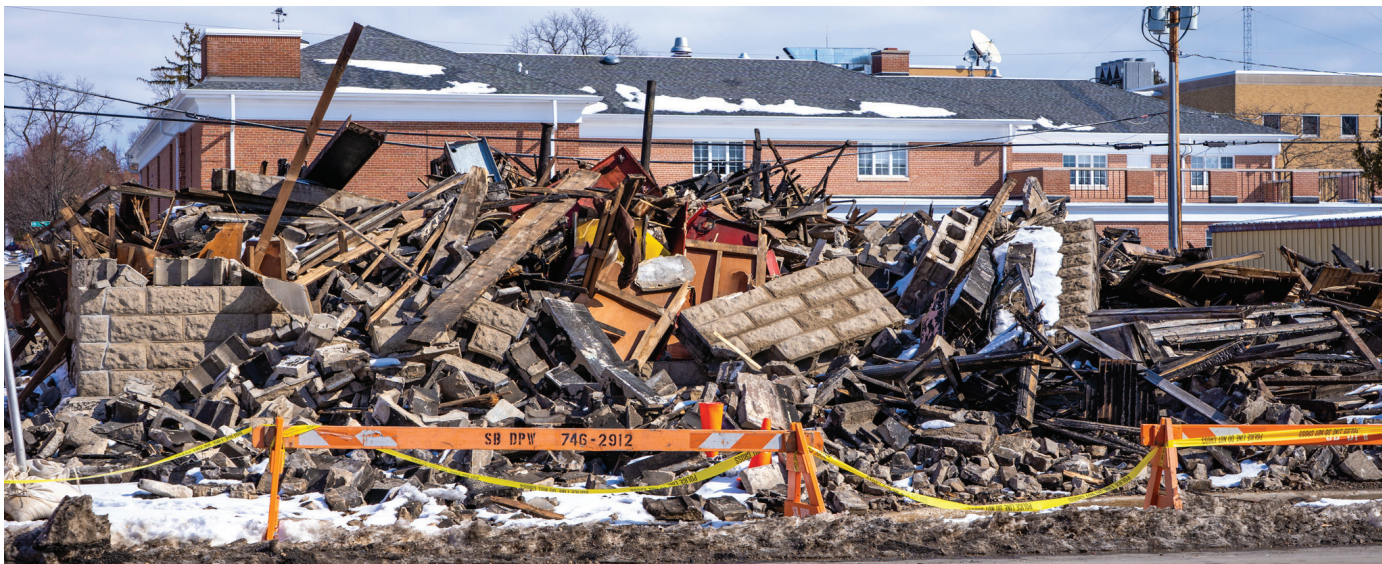
The demolition of the Butch's Bar building leaves a space on the corner of 3rd Avenue and Nebraska Street that has not existed since 1919, when the Butch's Bar building was constructed. The bodies of the two men who died in the Butch's Bar fire having been recovered, the building was demolished and reduced to a pile of rubble. Photo by Rachel Lukas.
