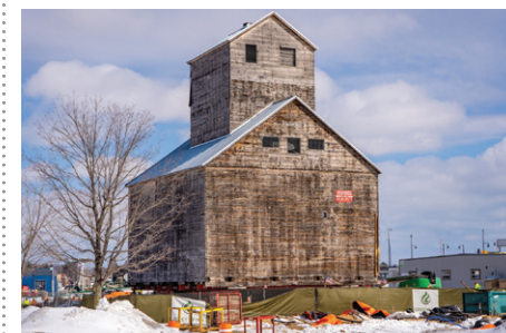
Work continues on the Door County Granary project on Sturgeon Bay's West Waterfront. Photo by Rachel Lukas.
