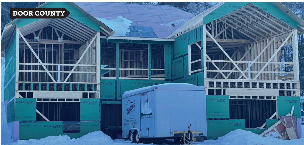
Existing housing stock sold quickly once it was on the market during the past two years, causing many buyers to scoop up land and go the route of building their own, such as this home under construction on Bay Shore Drive in Sevastopol. Photo by D.A. Fitzgerald.
