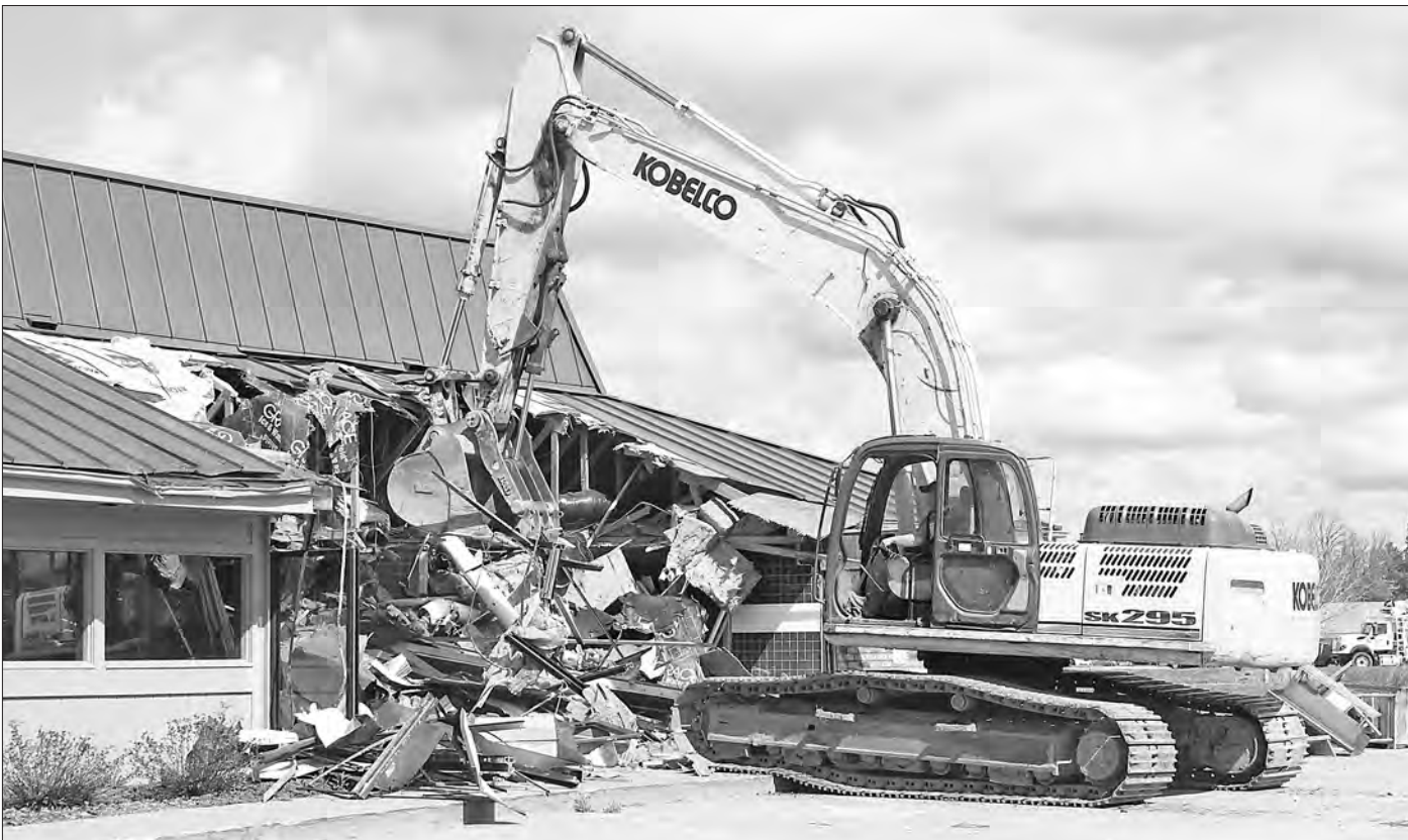
GOODBYE PIZZA HUT — Demolition began on the old Pizza Hut building in order to make way for the new Taco Bell that is coming
