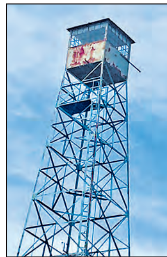
The fire lookout tower in Mosinee was one of 72 shut down by the Wisconsin Department of Natural Resources in 2016, when the fire-spotter program was eliminated after a century of service.
